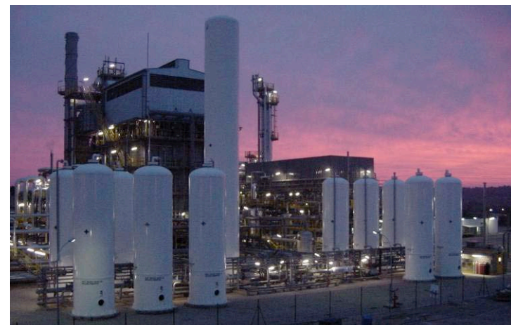
Air Products' 63 MMSCFD SMR enabled an European refinery to meet environmental regulations and growing diesel demand.
